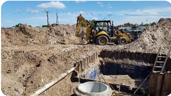
HCE's successful experience and knowledge of gravity sewer design and construction will benefit OUA on this project.
