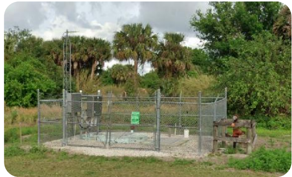
HCE will verify existing wastewater infrastructure and capacities
